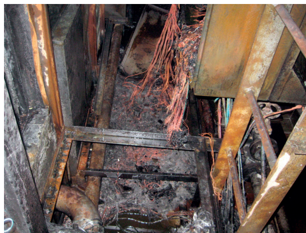
Figure 3. Part of an engine room after a fire (U.S. Coast Guard Newsroom, 2015)
